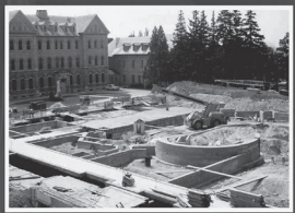
When the need for a new friary and auditorium arose, the architect Charlie Roe convinced the friars that he could build a more suitable chapel for the renewed liturgy as envisioned by Vatican II. Thus it was decided after only twelve years of use to convert the student chapel in St. Conrad Hall into an auditorium.
