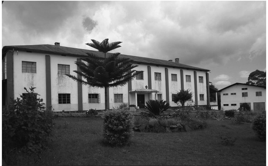
The Friary of the Seminary is aging and in need of a new roof.
